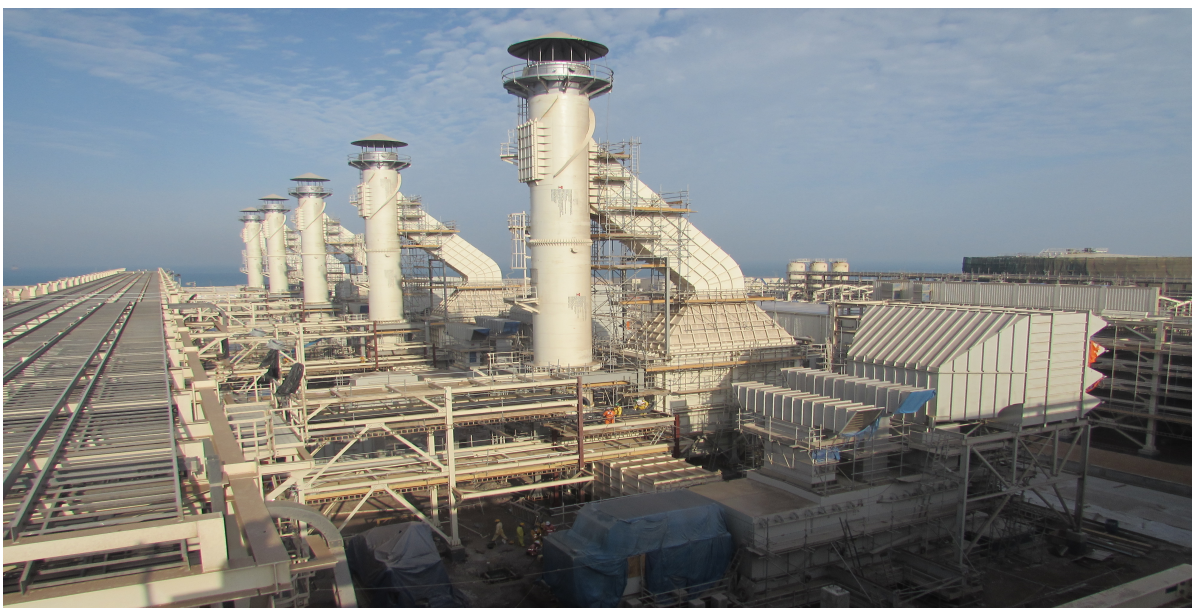
5 units of 36.19 mw waste heat recovery unit supplied to one of the renowned oil major in Abu Dhabi
