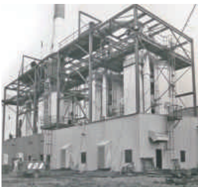
4 coil type boilers at Shell site in Canada, generating 33 TPH steam at 162 Bar pressure.
