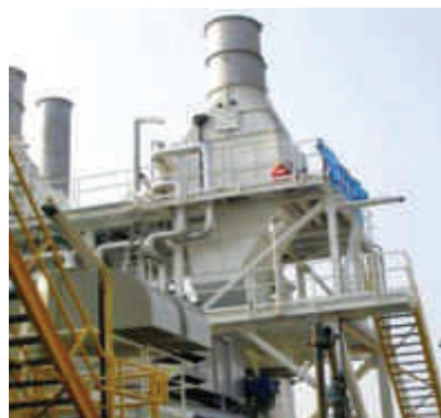
WHRU with a typical 2 stack design behind a gas turbine.
