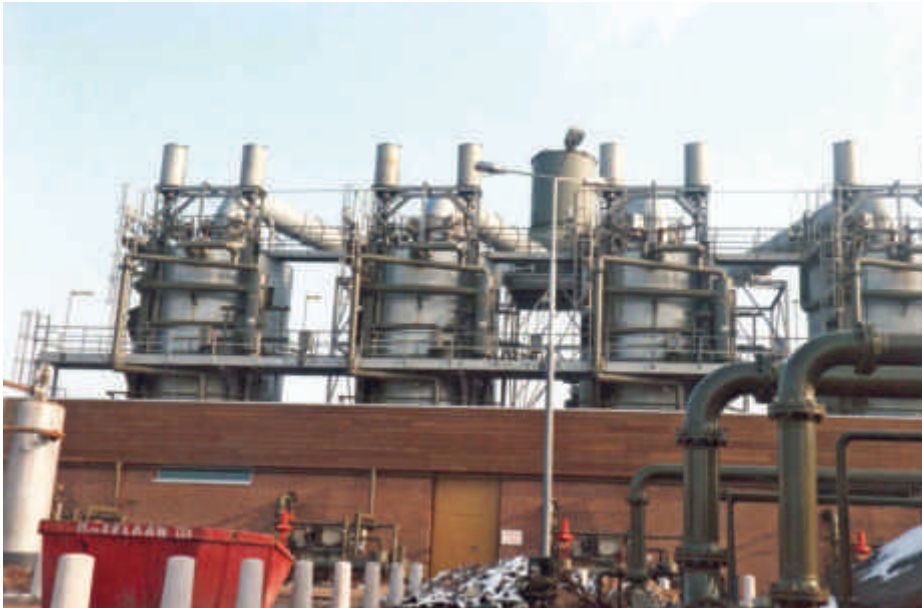
4 X 100 Mn Btu/Hr Once Through Steam generators at Shell project in Canada.
